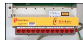
Figure 6: 7250BB-50 Break-Out Box installed on 720000 TeleLite Shelf
