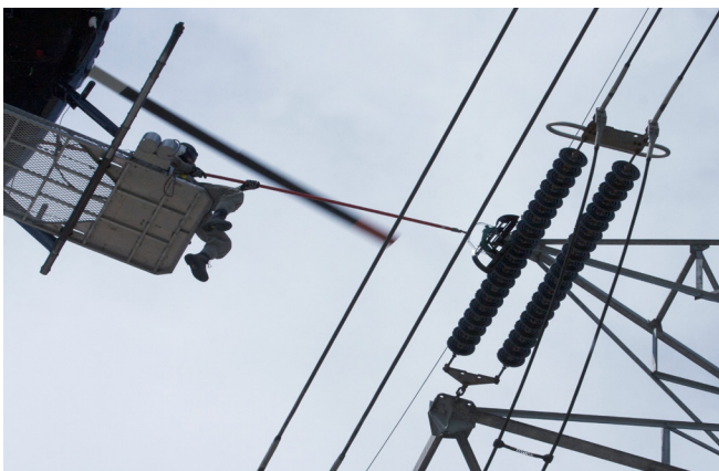
Testing Porcelain Insulators with a Helicopter
