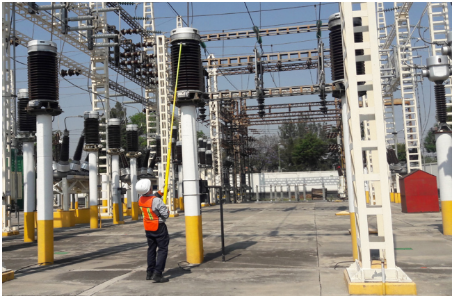
Testing Bushing Insulators in a Substation
